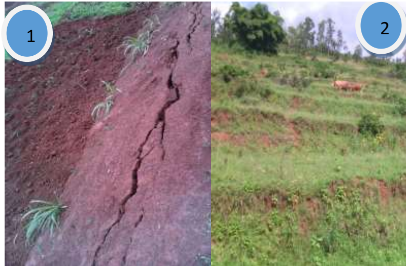
Plate 1. (1) The embankment started cracking few weeks after terracing, (2) abandoned terraces are actually used as pasture land Source: Field Data (2015)
